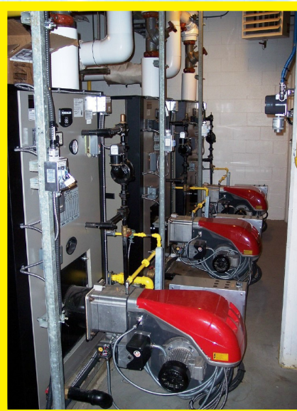
New boilers up and running in the Halifax WWTF-March 2010
