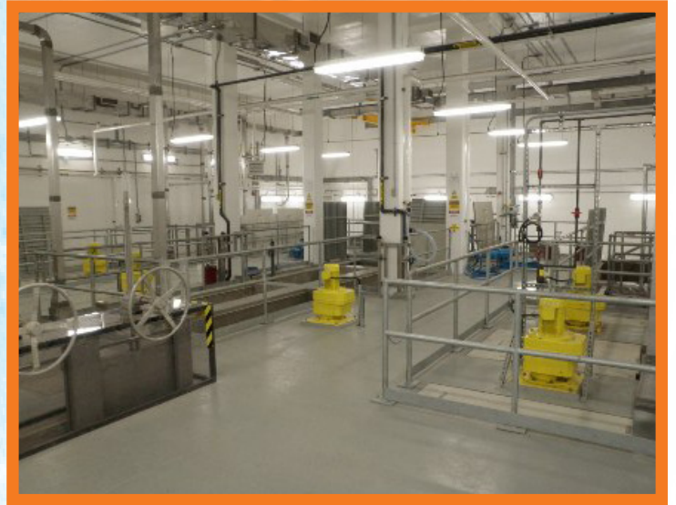
Densadeg wastewater treatment area
