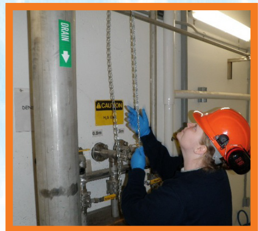
Katie MacDougall, Process Technician, performing system maintenance
