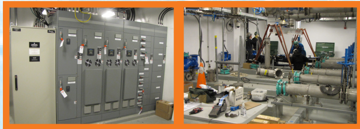
Crews working on new Motor Control Centre in basement of Halifax WWTF
