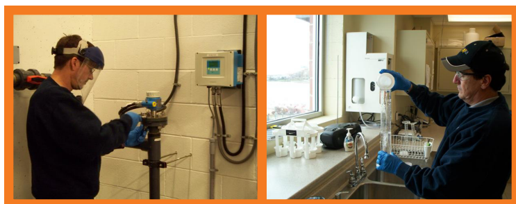
Mike Deagle, Process Technician, checking odour control system instrumentation
