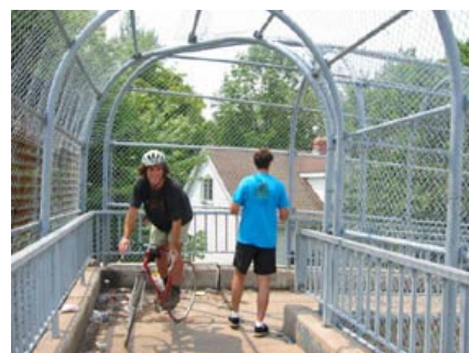
While the bridge is ramped, it is very narrow and has a number of extremely tight curves. Therefore, it does not meet spec for a shared use path. However, it is the only existing pedestrian access from Prince Albert to Main St. It is recommended that the bridge be used for one way cycle traffic only and that if it is upgraded that it provide a 4.0m wide path.
