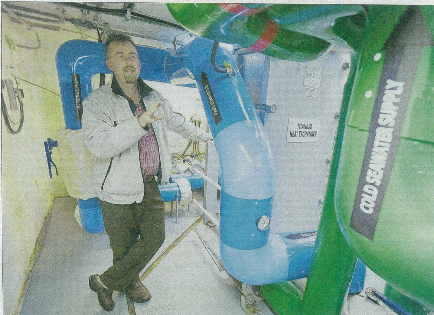
Julian Boyle, an engineer with Halifax Regional Municipality, displays the structure housing a geothermal system that will heat and cool Alderney Landing in Dartmouth. (CHRISTIAN LAFORCE / Staff)
