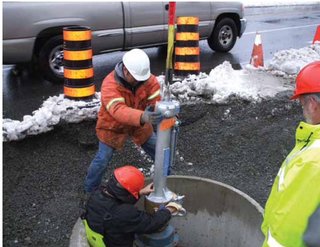
Launch of the “Pipe Diver” to assess water transmission main condition on Hammonds Plains Road
