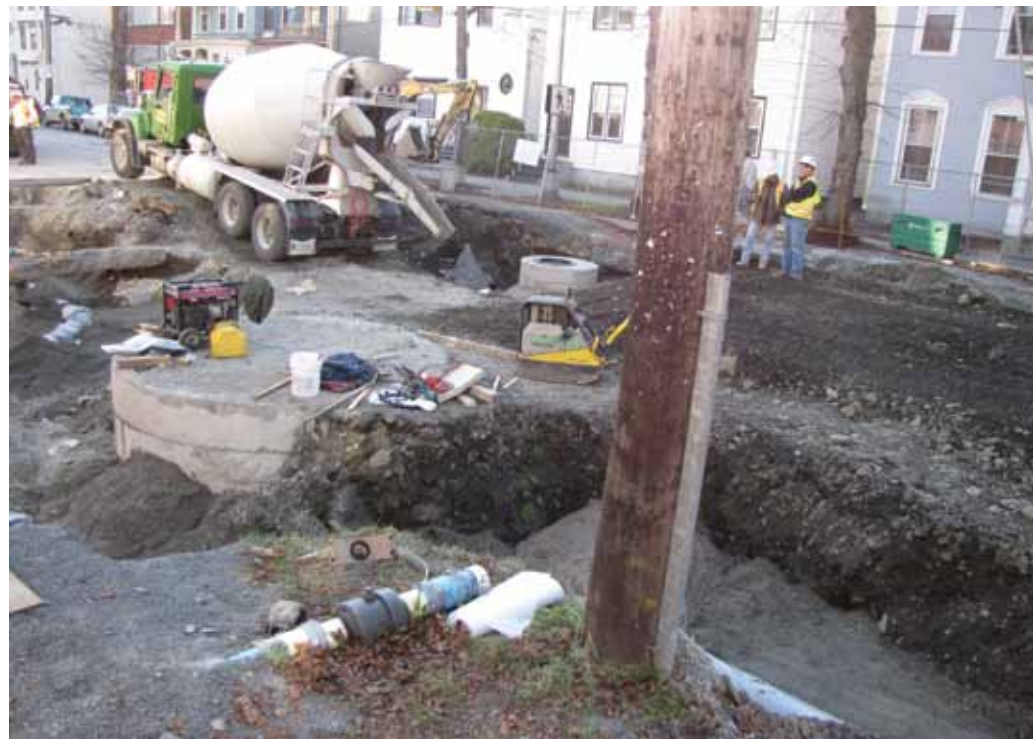
Below: Freshwater Brook Project at the intersection of Fenwick and South Park Streets
