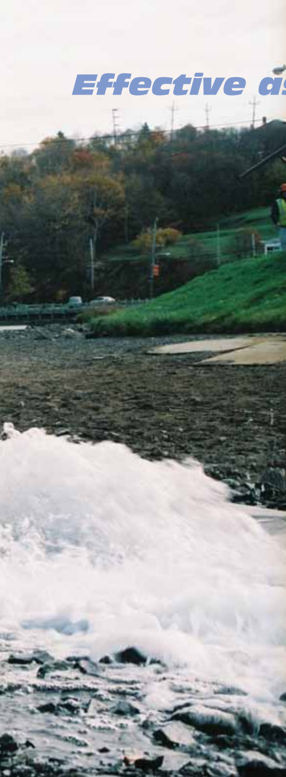
Above: Lowering of Lake Banook in preparation for the North Dartmouth Trunk sewer installation
