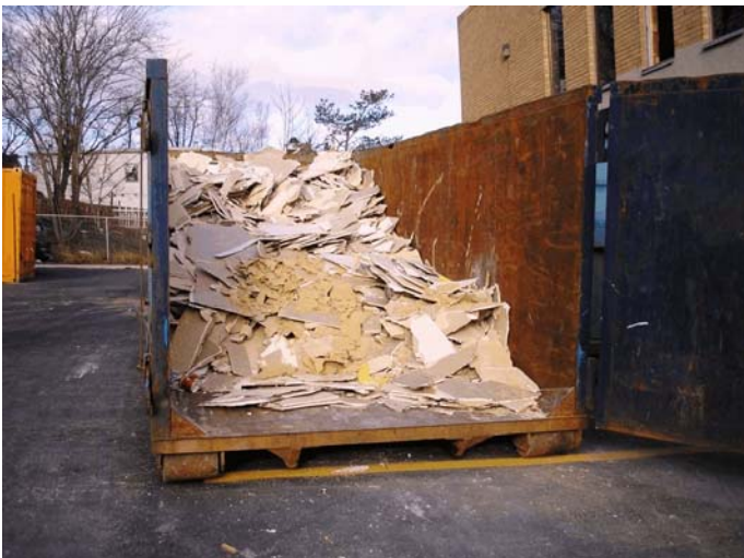
Having dedicated containers on site for sorting material saves time and disposal fees.
