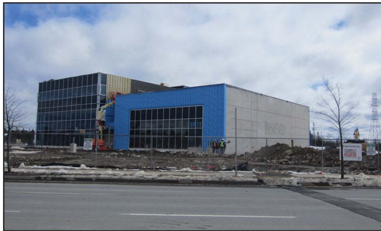
Progress is being made as construction continues for NSGEU at the corner of John Savage and Wright Avenue.
