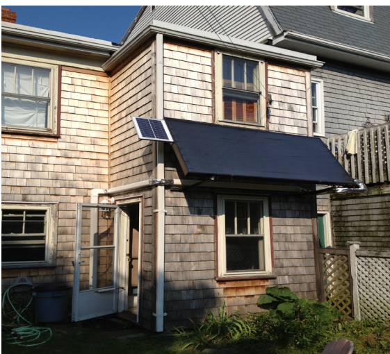
Solar hot water panel.
